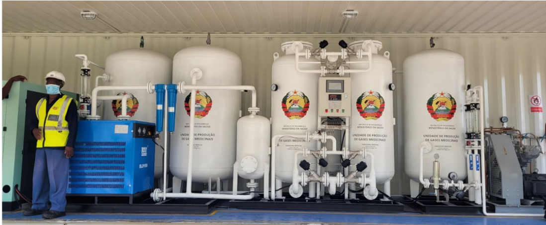
Figure 9. New PSA plant installed in the Nampula Central Hospital. (Picture: Marcello Passarana)
