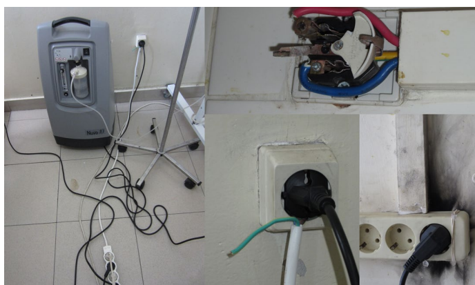
Figure 6. Examples of unsafe electrical connections (photos: Marcello Passarana)
